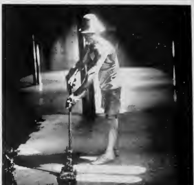
PITCHED in a shaft of sunlight pouring through a hole in the top, a workman spreads asphalt on the floor of a tank now being built on Serre Pretot. Soon this floor will be covered by 1,500,000 gallons of water.
